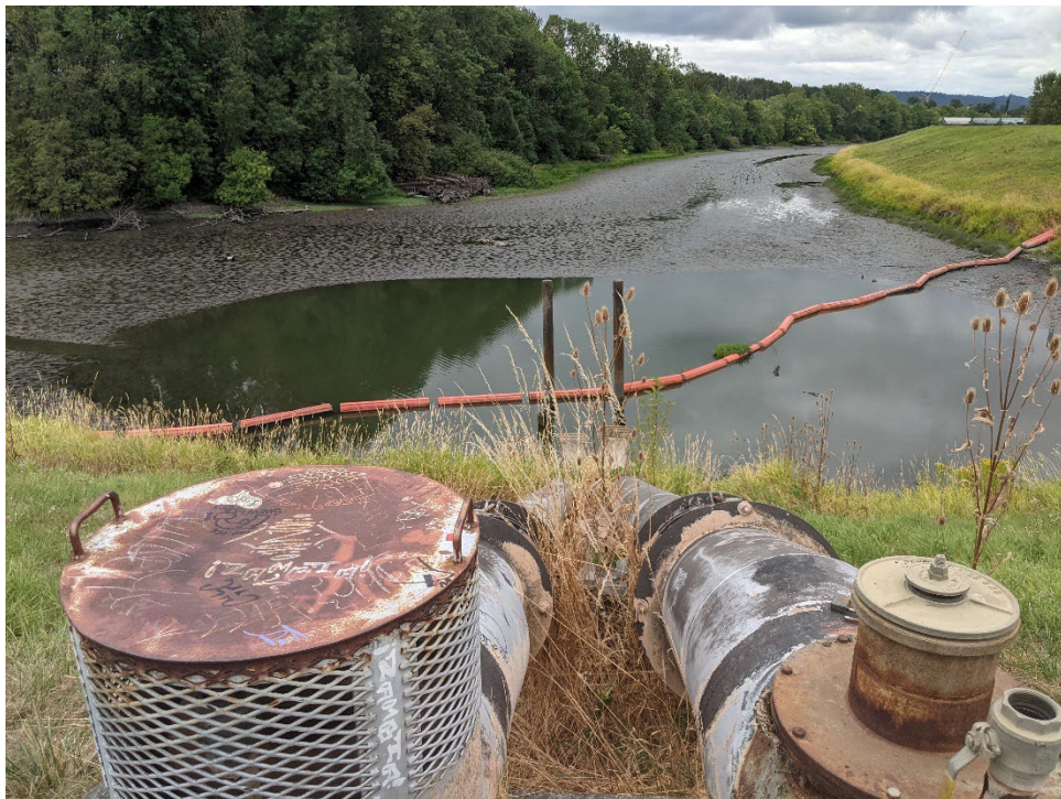
Photo 6. PIR Discharge into Columbia Slough
