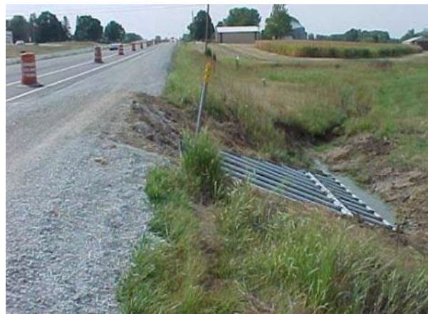
Photograph 7-1. Example of passive debris barrier at large culvert
